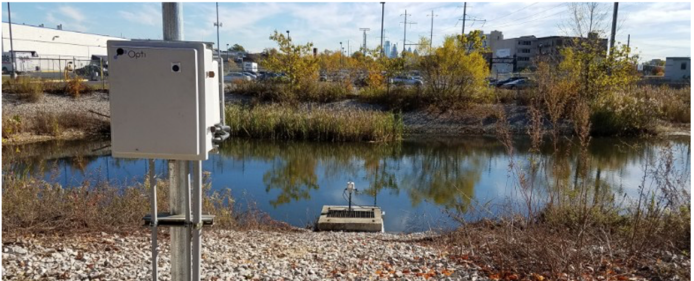
Opti's Smart Stormwater Management System
